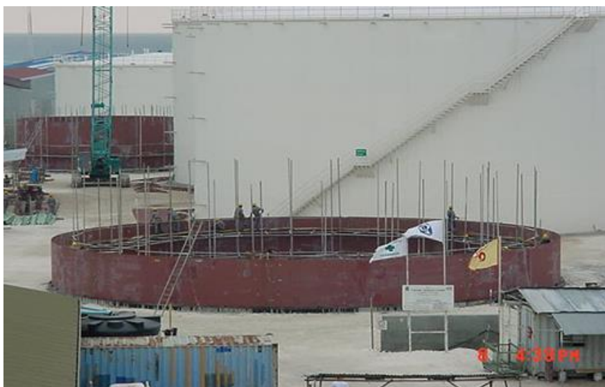
Petroleum Tank Farm in Maldives
