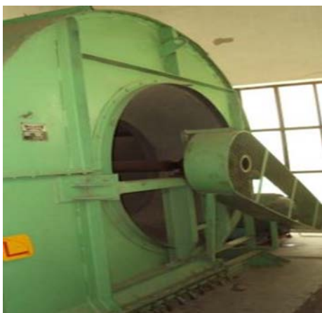
Blower & Control panel
