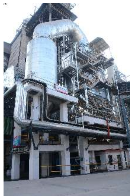
Waste heat recovery (WHR) is one of the key levers identified in the technology roadmap - WHR boiler
